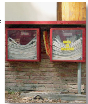
Current Fire hose station
