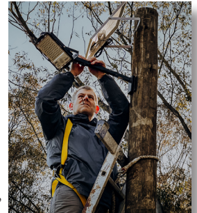
One of Jeff’s wiring jobs
