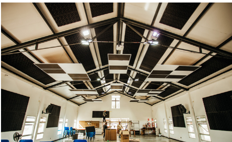
All the black panels are new acoustic tiles. Many more were added after this photo.
